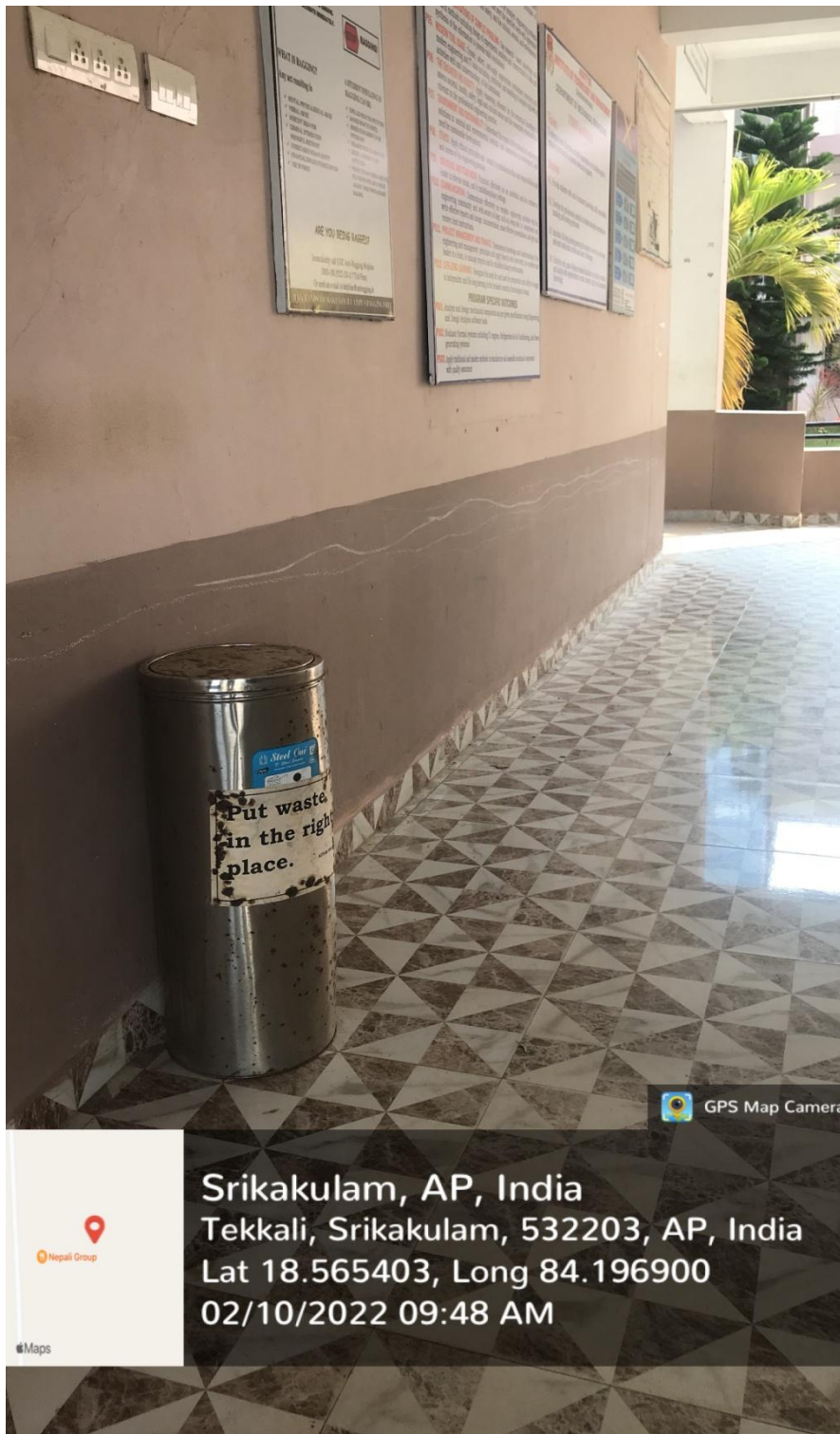
Common dust bin Installed in Ground Floor at 'E' Block (Sample)
