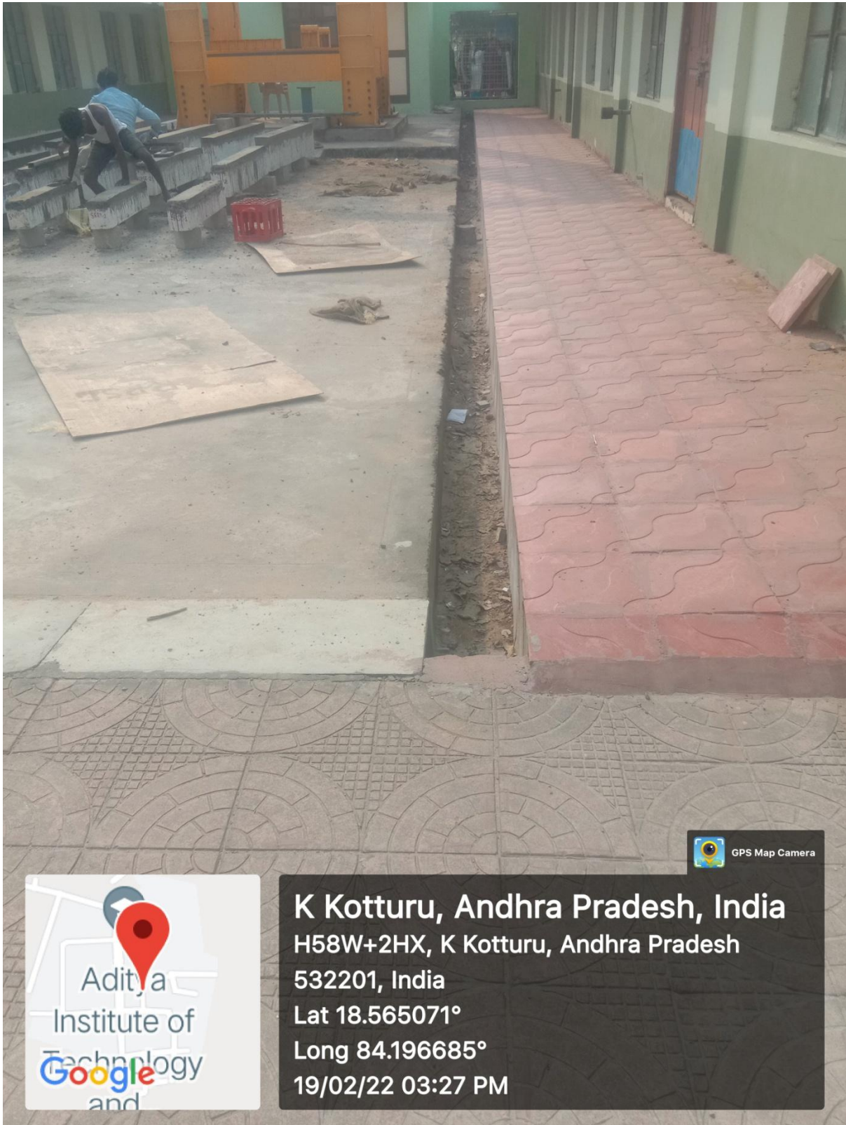
Sub drain for storm water collection
